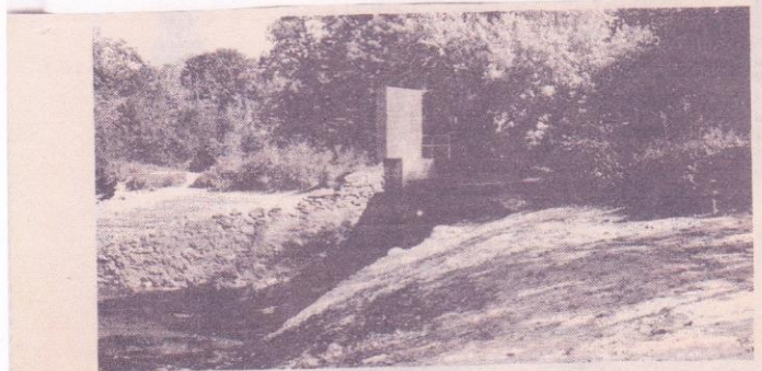
NOT ENOUGH SPILLWAY CAPACITY is the problem with the Gilman Brothers' dam at drained Lake Williams. The DEP has ordered the brothers to either repair or remove the dam. Photo by Lisa D. George
