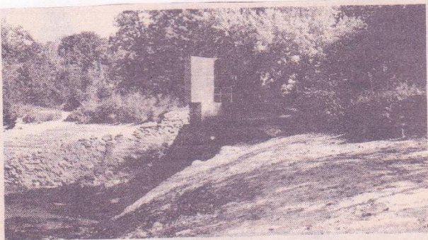
NOT ENOUGH SPILLWAY CAPACITY is the problem with the Gilman Brothers' dam at drained Lake Williams. The DEP has ordered the brothers to either repair or remove the dam. Photo by Lisa D. George
