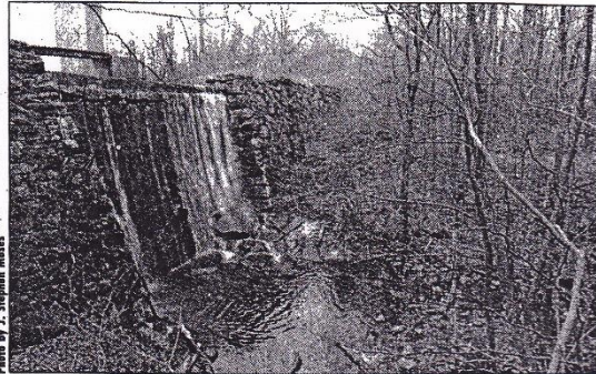
THE LAKE WILLIAMS DAM continues to deteriorate as state and town officials wrestle with a trouble-plagued plan for the state to take over the property.
